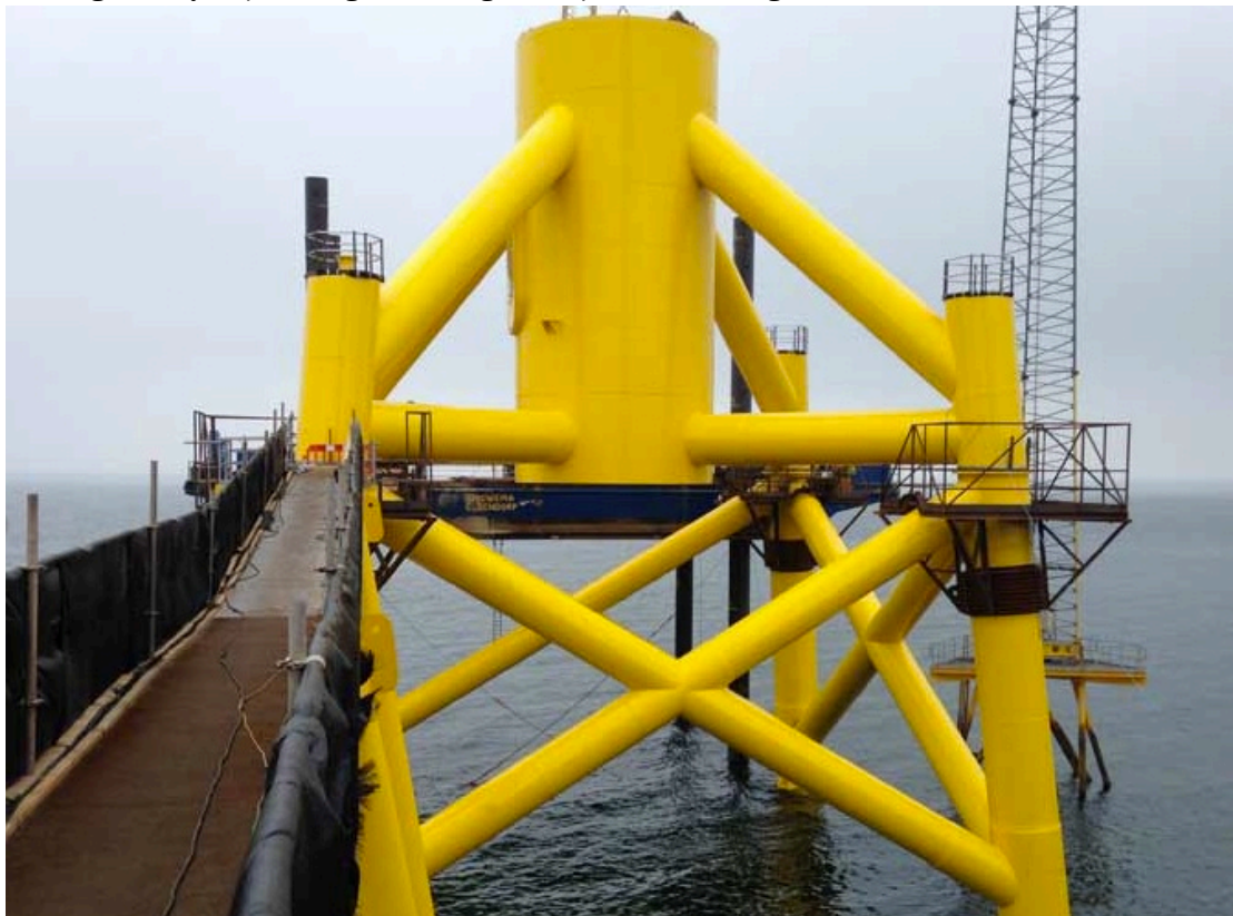
Figure 6.1-5: Simple strut model with external platform to be placed on top of the TP chords [Fife Jacket]
