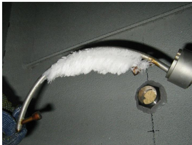
Figure 4.6: Ice build-up on non-heated spinner anemometer sonic sensor
